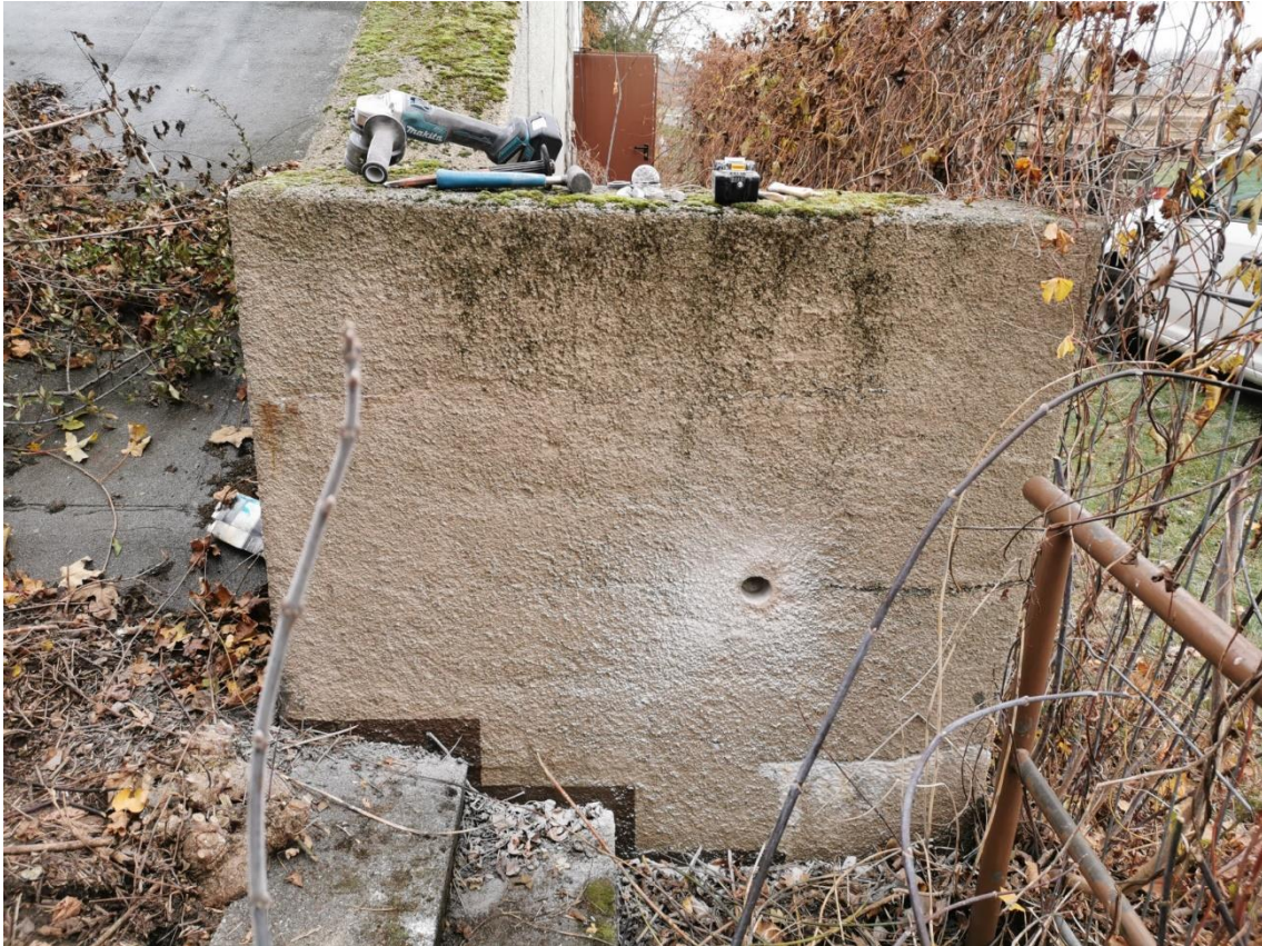
M6/ Horizontaler Riss
